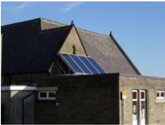
Solar thermal panels at Bradshaw Primary School
