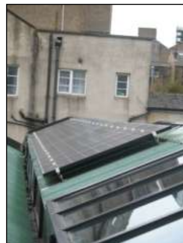
Solar PV panels at Sowerby Bridge Market
