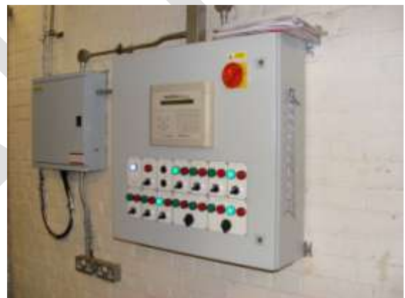
Advanced heating controls at Whitehill Community Primary School in Halifax
