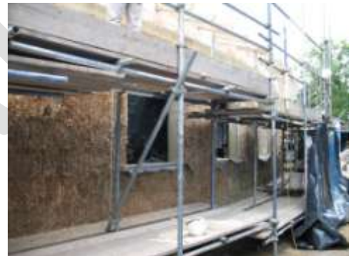
Shelf village hall extension – the walls are constructed of load-bearing straw bales
