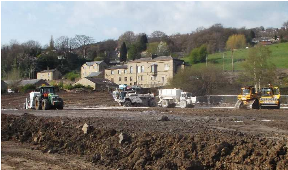
Plant working in the residential area to build up the site level
